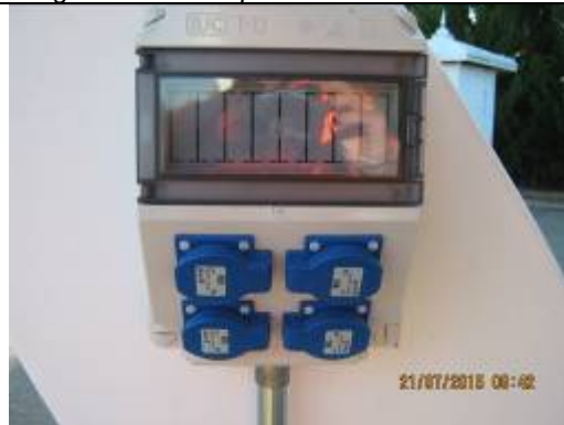
Image: Covered 230V 50Hz power outlet in workbench.
